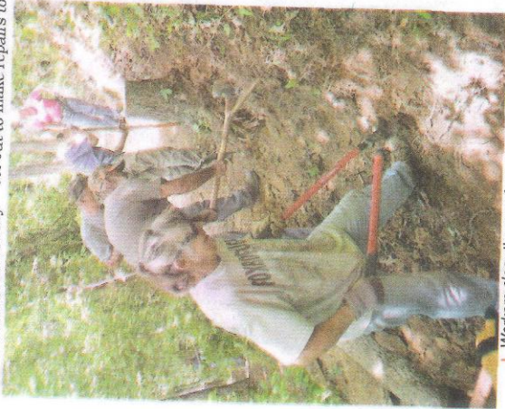
Workers clear the way for a wider and safer trail. Photo by Nancy Sluys
